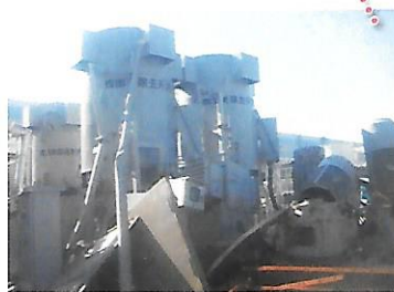
Seawater pump damaged by tsunami
